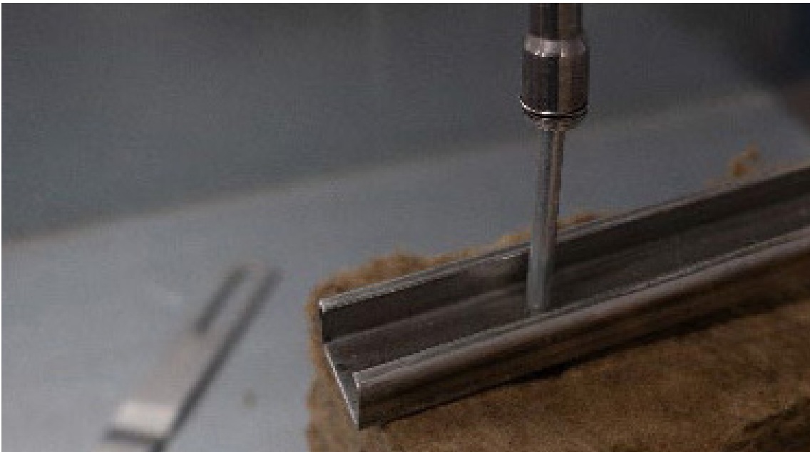
Figure 10 – Installation of fasteners for retention of wall-tie system to mild structural steels
